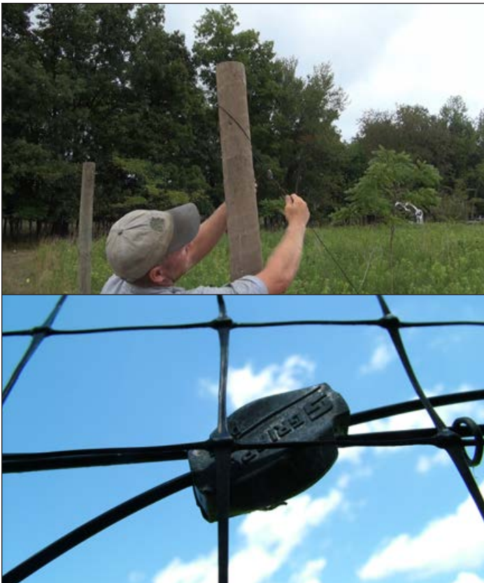
Figure 6. Secure the top monoline through a fence staple and attach a gripple.
