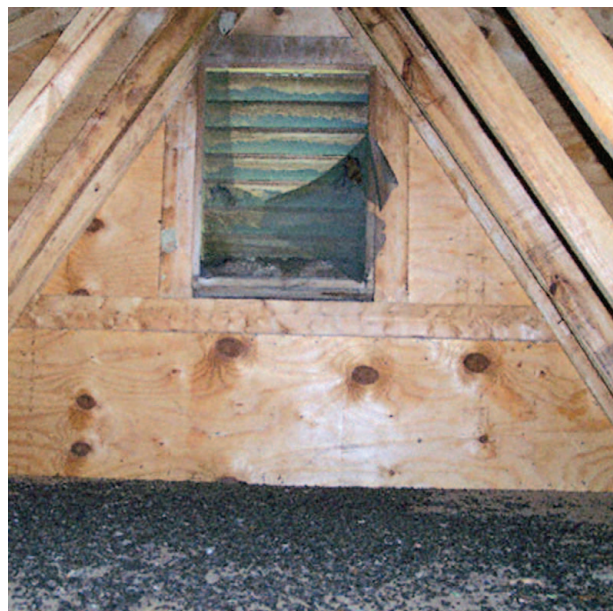
Bat guano in attic with damaged screen.
