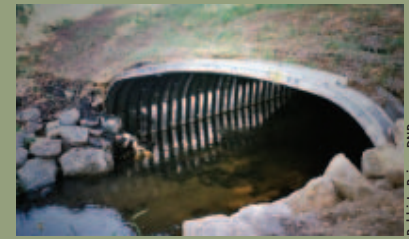
Structural plate-arch culverts are set in concrete footings, leaving the natural streambed almost entirely unchanged.
