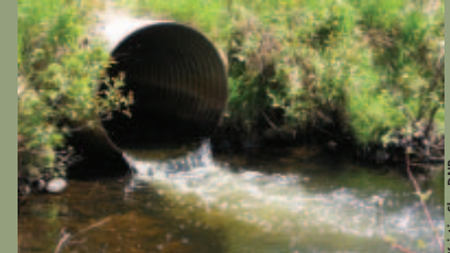
This culvert is perched. When culverts are perched, fish cannot enter it and will not be able to reach important segments of the stream.
