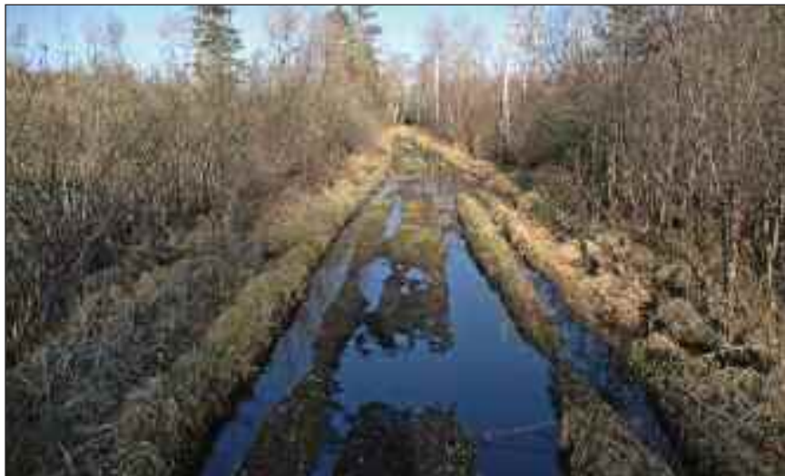
ABOVE: Wetland road needing repairs to protect wetland and support traffic
